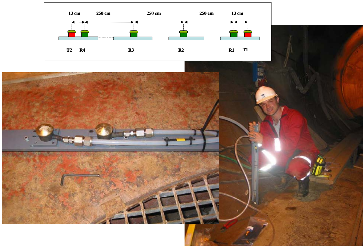
Figure 3-1: Top: Schematic diagram of the locations of all transducers on a single frame. Left: Photo of a section of the transducer assembly. Right: The transducer assembly during installation.
